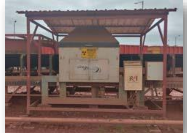
RTI's AllScan cf-252 elemental analyser on site.
